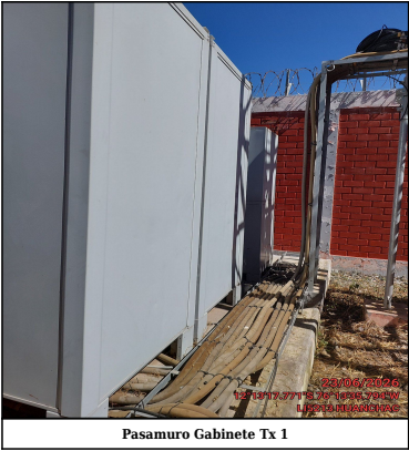
Pasamuro Gabinete Tx 1
