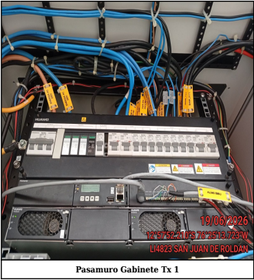
Pasamuro Gabinete Tx 1
