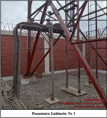
Pasamuro Gabinete Tx 1
