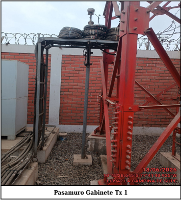
Pasamuro Gabinete Tx 1
