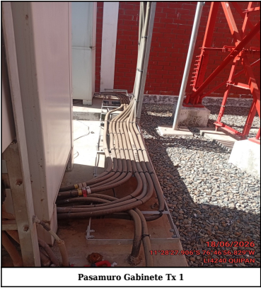
Pasamuro Gabinete Tx 1
