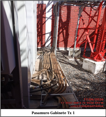
Pasamuro Gabinete Tx 1
