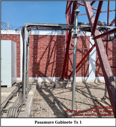
Pasamuro Gabinete Tx 1
