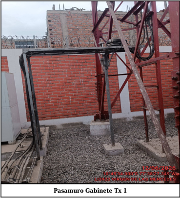
Pasamuro Gabinete Tx 1
