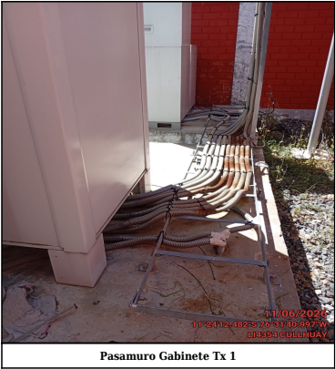
Pasamuro Gabinete Tx 1
