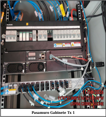
Pasamuro Gabinete Tx 1
