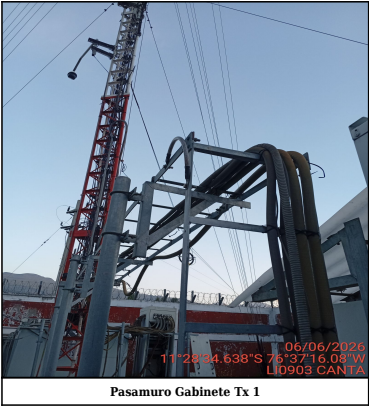
Pasamuro Gabinete Tx 1
