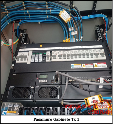
Pasamuro Gabinete Tx 1
