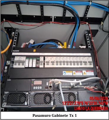
Pasamuro Gabinete Tx 1
