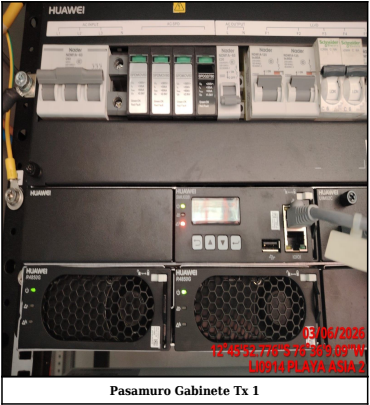
Pasamuro Gabinete Tx 1
