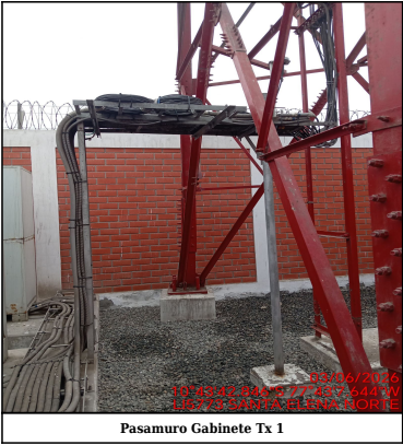
Pasamuro Gabinete Tx 1
