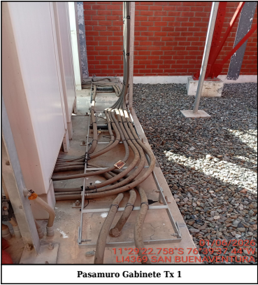
Pasamuro Gabinete Tx 1
