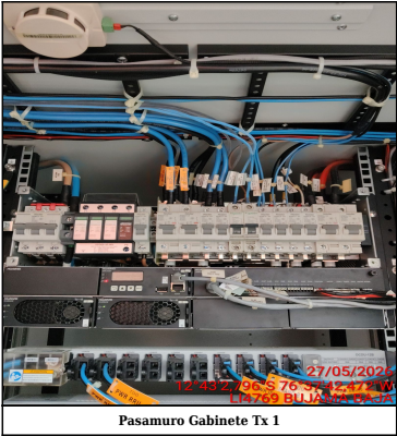
Pasamuro Gabinete Tx 1
