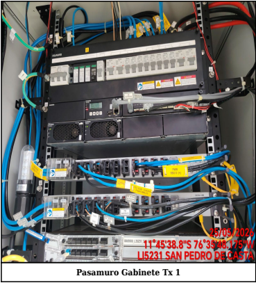
Pasamuro Gabinete Tx 1
