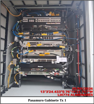
Pasamuro Gabinete Tx 1
