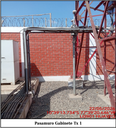
Pasamuro Gabinete Tx 1
