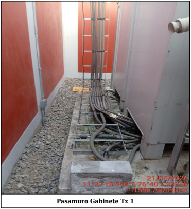
Pasamuro Gabinete Tx 1
