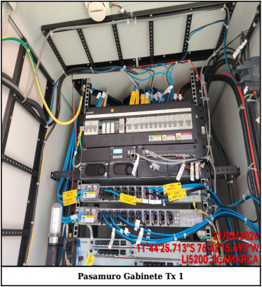
Pasamuro Gabinete Tx 1
