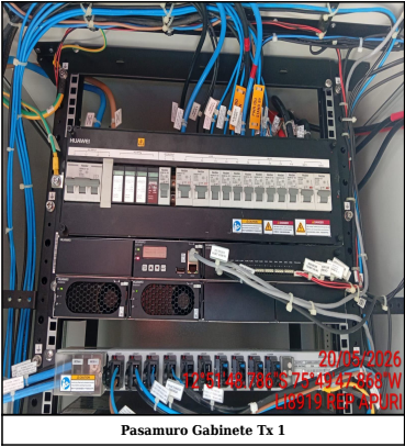
Pasamuro Gabinete Tx 1
