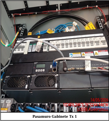
Pasamuro Gabinete Tx 1
