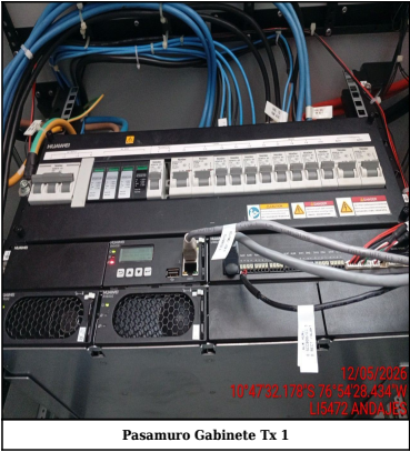
Pasamuro Gabinete Tx 1
