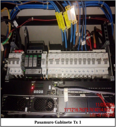
Pasamuro Gabinete Tx 1
