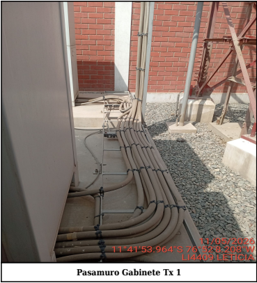
Pasamuro Gabinete Tx 1
