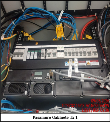
Pasamuro Gabinete Tx 1
