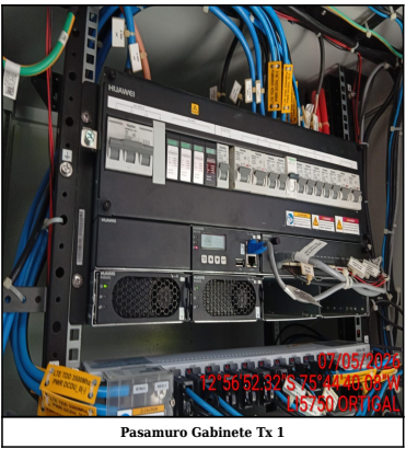
Pasamuro Gabinete Tx 1
