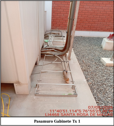
Pasamuro Gabinete Tx 1
