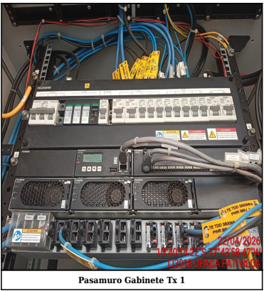
Pasamuro Gabinete Tx 1
