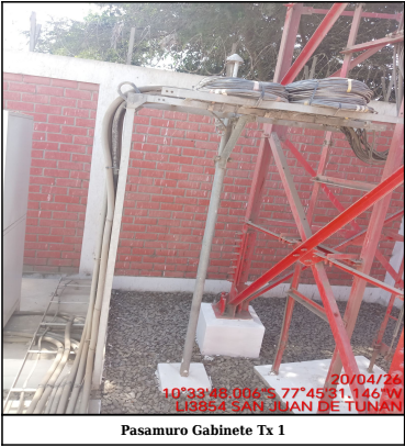
Pasamuro Gabinete Tx 1
