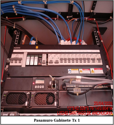
Pasamuro Gabinete Tx 1
