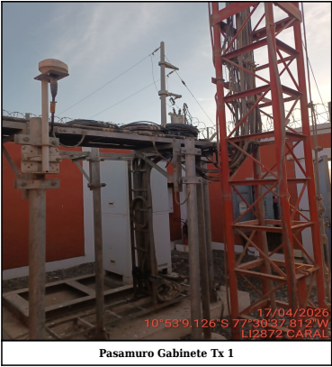
Pasamuro Gabinete Tx 1
