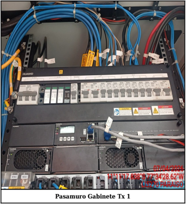
Pasamuro Gabinete Tx 1
