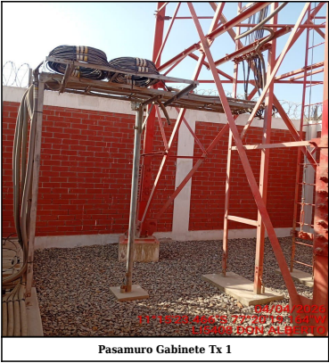
Pasamuro Gabinete Tx 1
