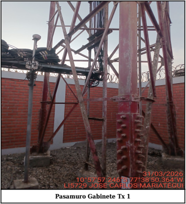
Pasamuro Gabinete Tx 1
