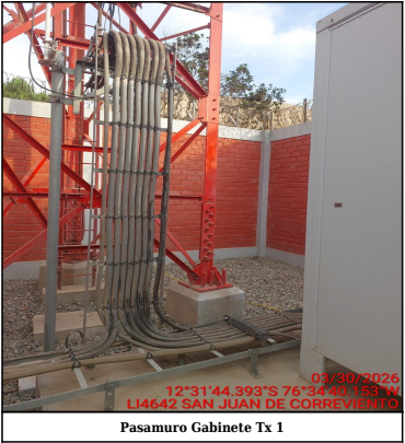
Pasamuro Gabinete Tx 1
