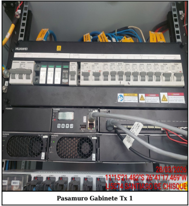
Pasamuro Gabinete Tx 1
