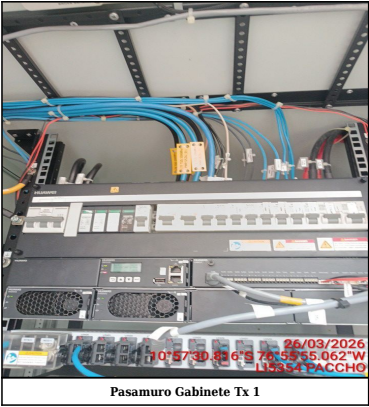
Pasamuro Gabinete Tx 1
