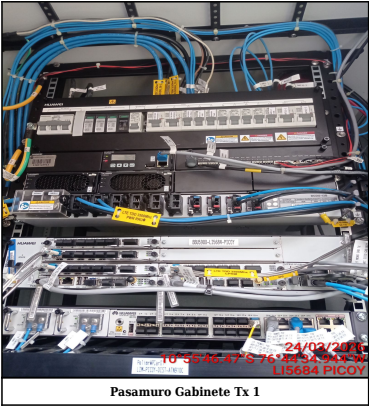
Pasamuro Gabinete Tx 1
