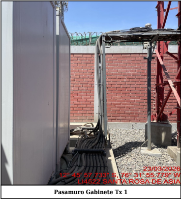
Pasamuro Gabinete Tx 1
