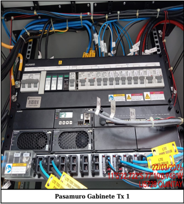
Pasamuro Gabinete Tx 1
